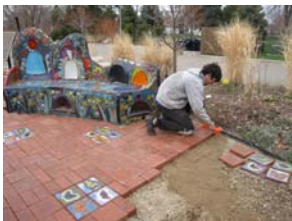
Caption: Travis Borowicz of J.T. Earthworks installs personalized pavers near the butterfly art bench in the Great River Road Learning Center's butterfly garden. Photo by Margaret Smith
